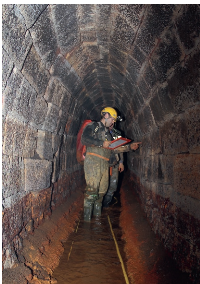
Fig. 8. Elliptic gallery lining of sandstone blocks between the 807.1 and 810.1 m marks. The masonry blocks in the left sidewall have been pushed in; view looking to the south east.
